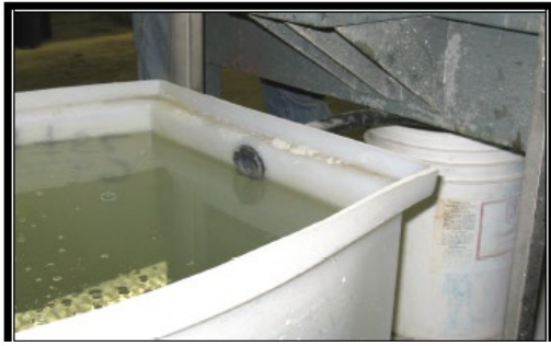
Figure 3: Water overflow outlet
